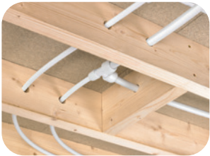
Easy cabling. Fewer joints
