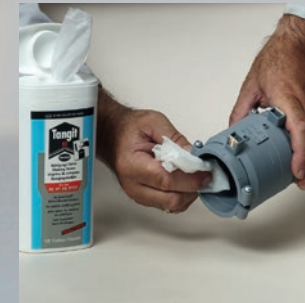
Clean pipe and fitting
