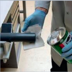
Clean pipe and fitting
