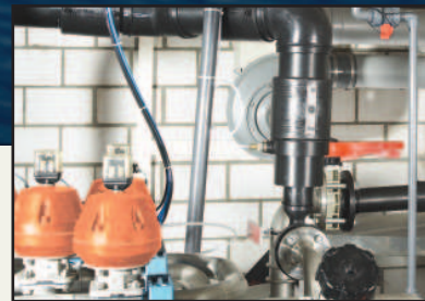
Industrial Wastewater Treatment
